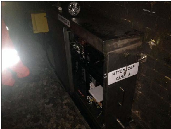
Location case with door missing
